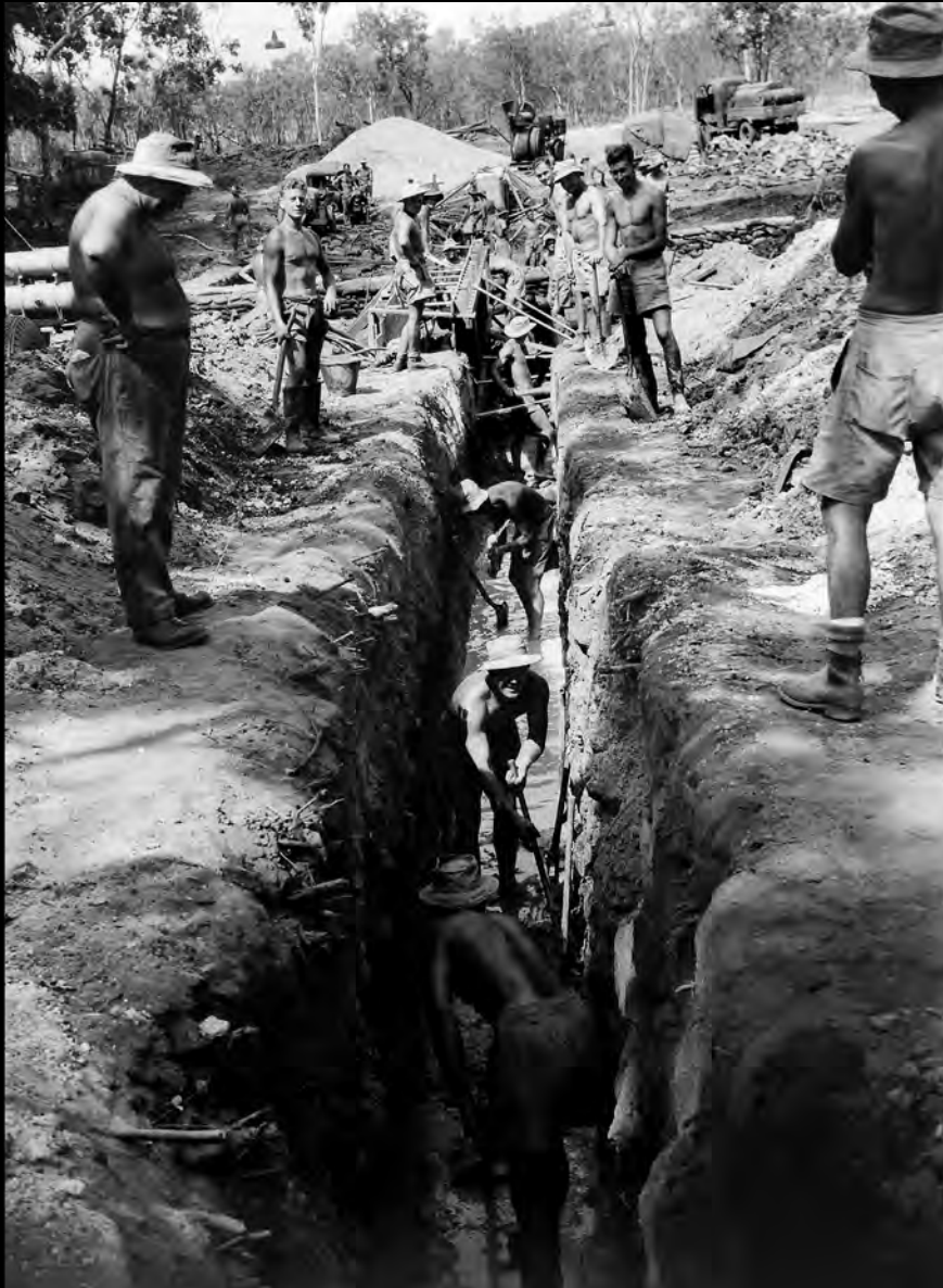
Members of the 1st Field Company, Australian Engineers, excavate a pipeline during construction of a weir to dam water for elevated tanks at Paraparap, Howard Springs, September 1944. (AWM 081111)
